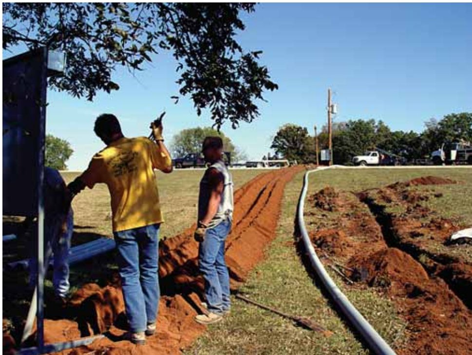
IEC donated the electric line which City of Cleveland contractors laid underground for the Country Fest celebration in October at Feyodi Recreation Area.
